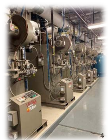
Heating and Cooling Systems
