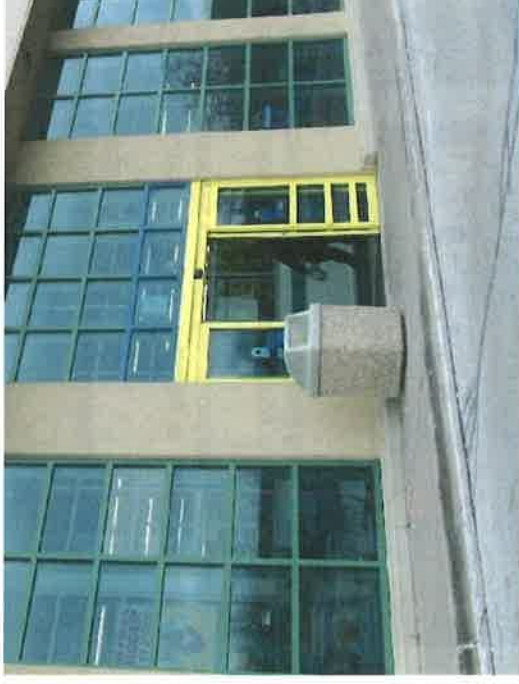
Discouraged: Featureless, window-dominated entranceway.
