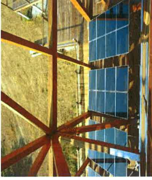
Solar panels incorporated into building elevation/roof top.
