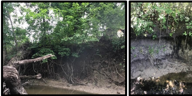
Figure 4. Examples of severe erosion along stream banks.
