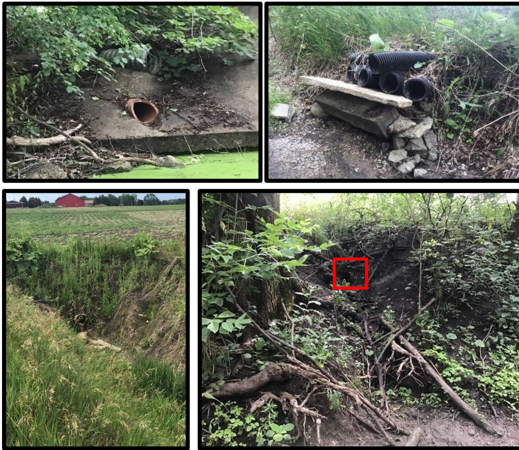
Figure 9. Examples of functional discharge points: clay tile (top left), HDPE (top right). Examples of problem discharge points, where outflow from damaged pipes is creating erosion along stream banks: clay tile (bottom left) and ductile iron (bottom right).
