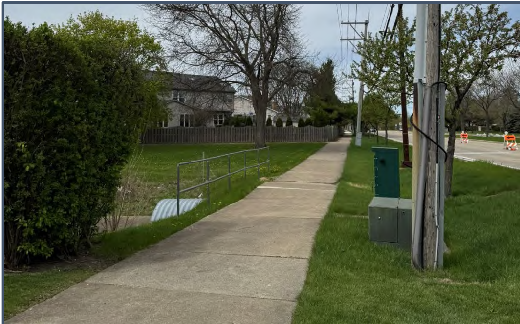
Photograph 2–Looking over Culvert (dip in Sidewalk)
