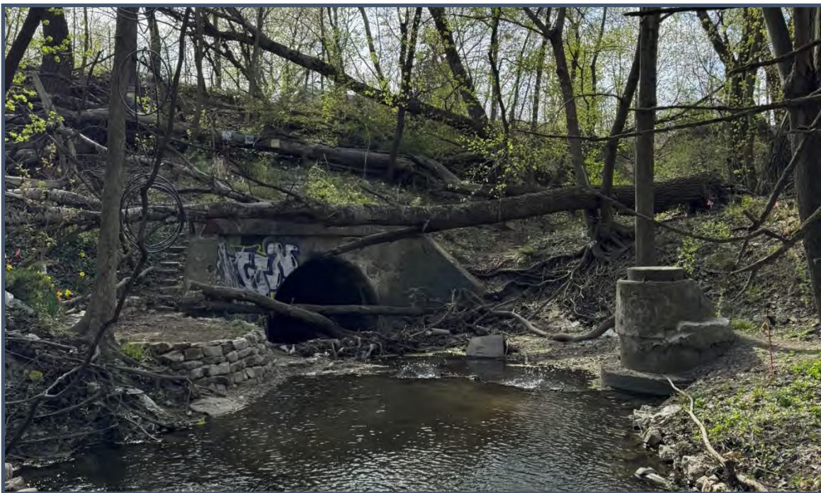
Photograph 2- West Elevation, Scour at Drainage structure
