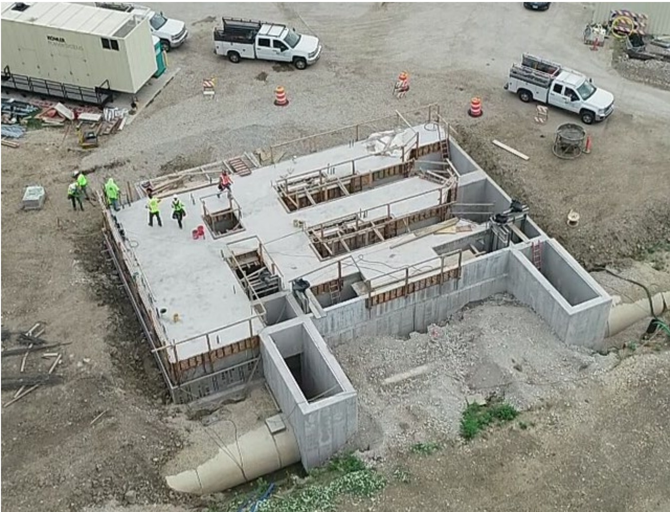
DPR WRF UV Disinfection Improvements
