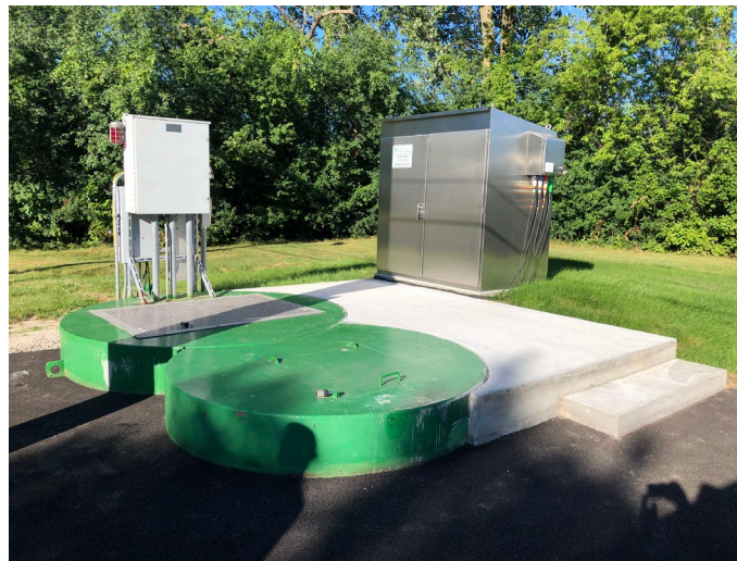
Figure 2- Typical Post-Improvement Site - Electrical/Control Enclosure
