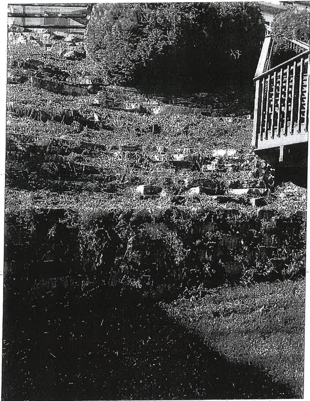
Subject property showing deterioration of prior retaining wall
