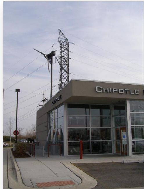
Building-mounted wind turbine
