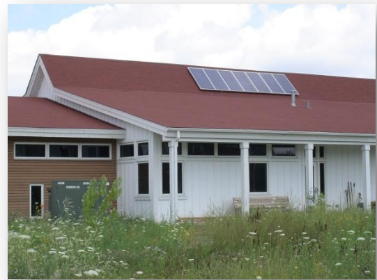
Building-mounted solar panels
