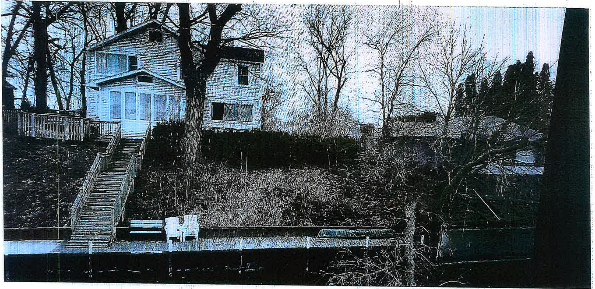
View of property two homes east of subject property showing erosion and loss of mature trees
