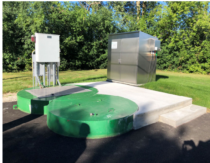
Figure 2- Typical Post-Improvement Site - Electrical/Control Enclosure
